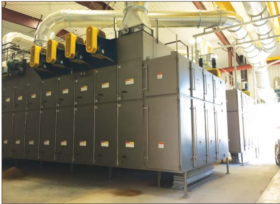
Two Buhler Aeroglide dryers replace conventional pellet coolers at the Ainsworth mill. They are designed to increase range cube shelf life by removing all water activity. Photo courtesy of EBM Construction Inc.
